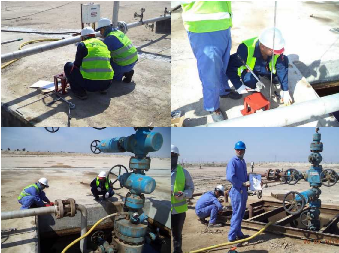
(Pilot device detector installation)
