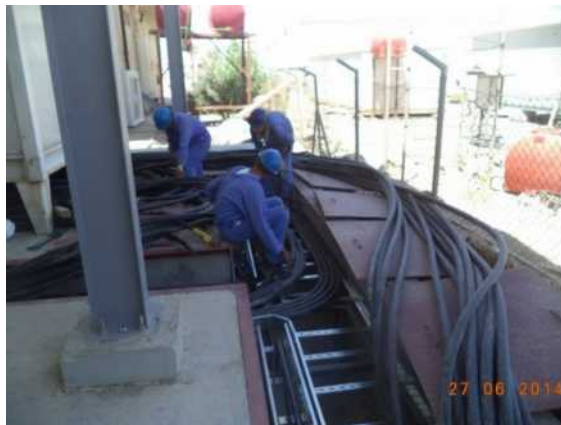
(Cable transformation kit of generators & TRF.)
