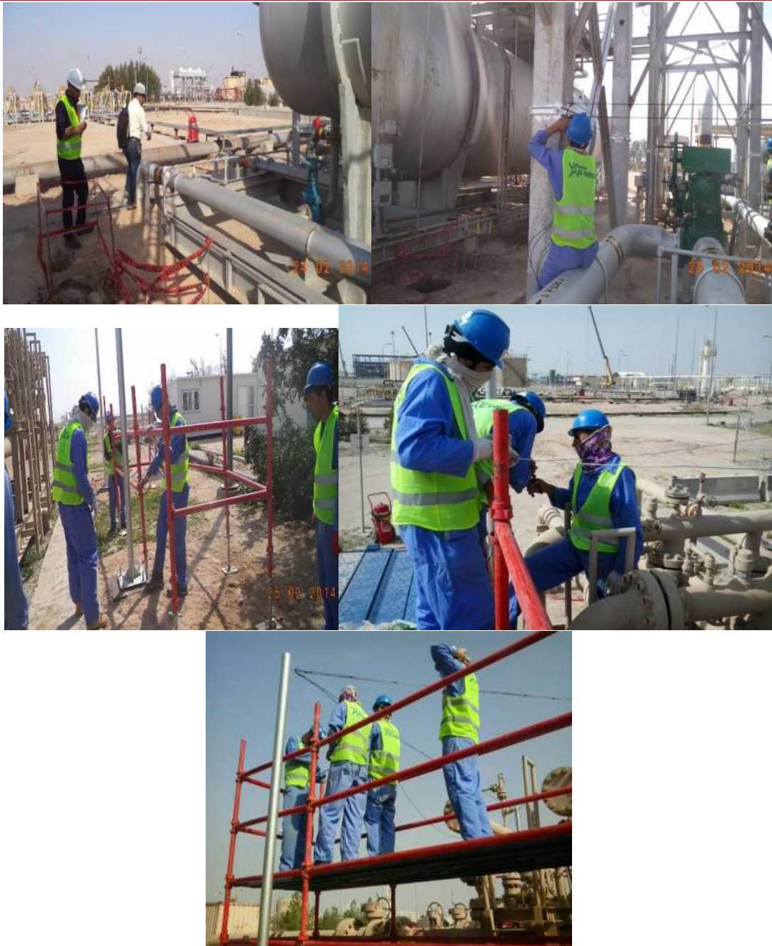
(Linear heat detector (LHD) installation)
